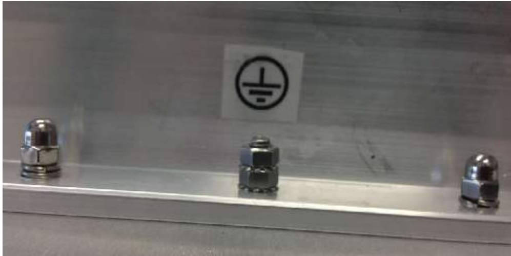
Figure 44: 9502 Protective earth grounding
