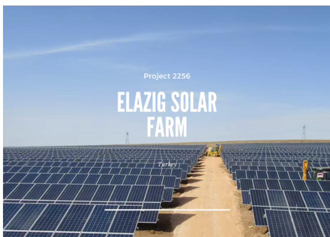
Project 2256: Elazig Solar Farm in Turkey
