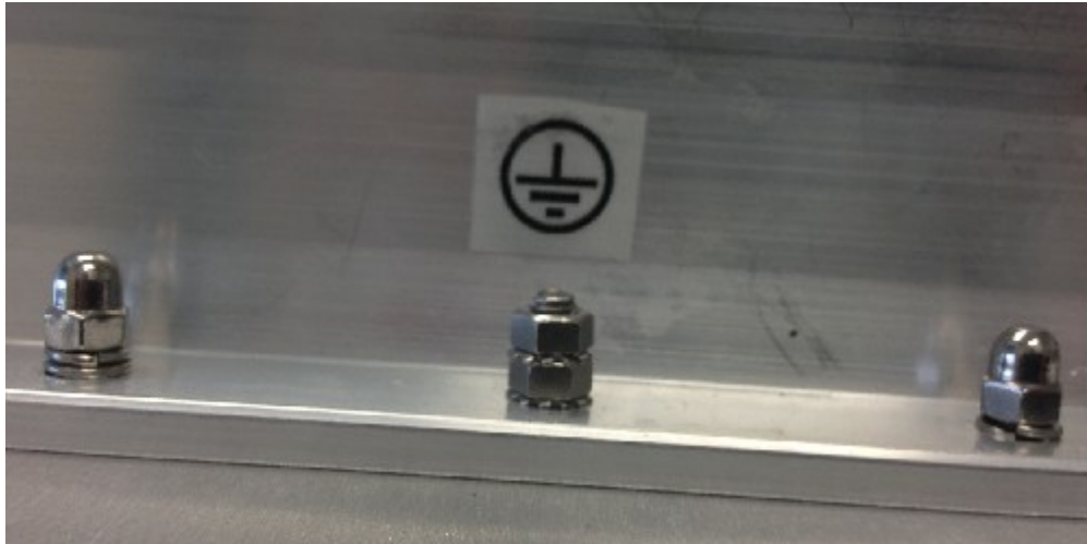
Figure 46: 9502 Protective earth grounding
